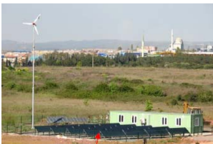
Figure 8: The HYDEPARK Photovoltaic field and wind turbines [13]
